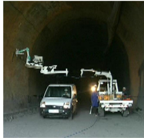
Figure 15. TunConstruct system test in a Spanish tunnel. Note that one lane of the tunnel traffic flow is not blocked
