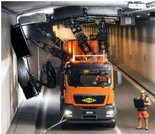
Figure 10. Tunnel cleaning system [55]
