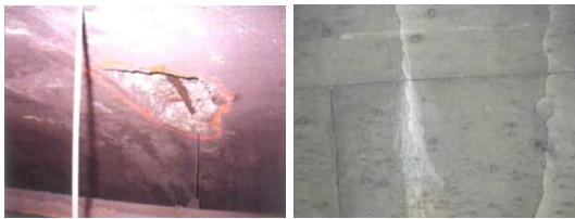
Figure 2. Examples of spalling (left) and crack with efflorescence (right) [5]
